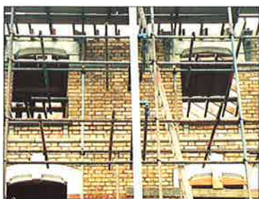
Rehab development of a derelict property purchased from London Borough of Hackney for conversion
